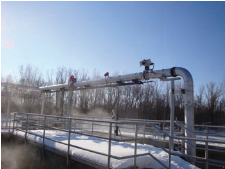
Stainless steel piping delivers air from blowers to aeration basins.
