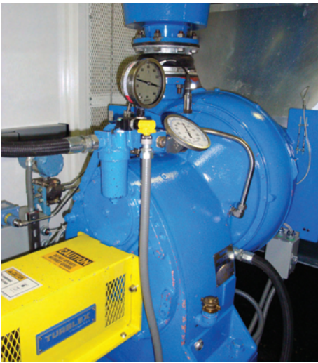
One of three energy efficient variable vane blowers installed.
